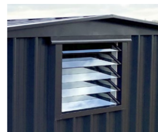
Louvre window allows natural light and airflow.
